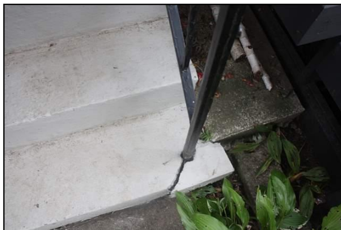
10. Masonry or concrete cracking
