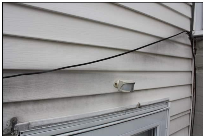
5. Loose or missing pieces
