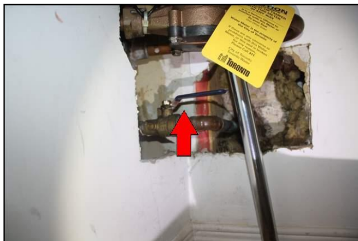
20. Main shut off valve
