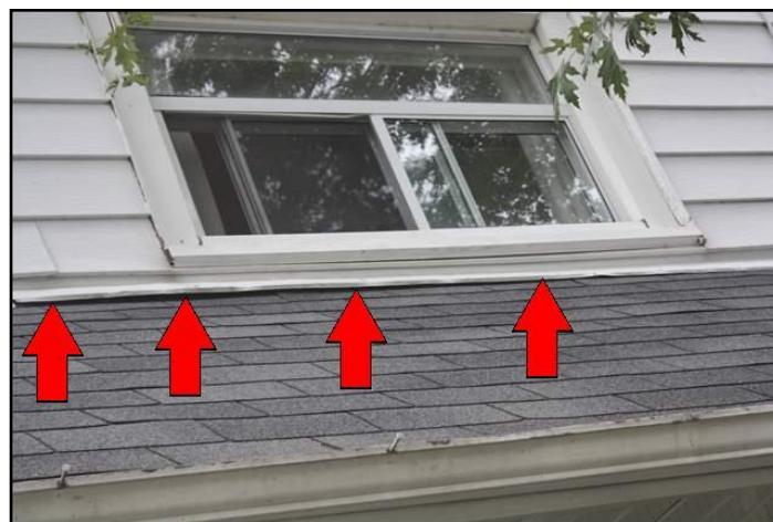
1. Damage, loose, open seams, patched
