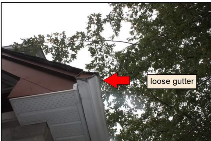
2. Aging - Wear and tear noted. Fasteners...
