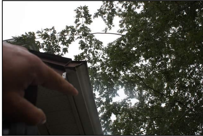
13. Trees or shrubs too close to building
