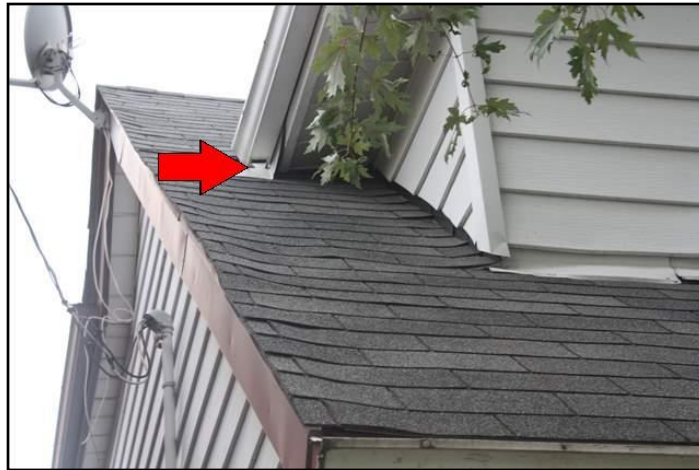
4. Discharge onto roofs
