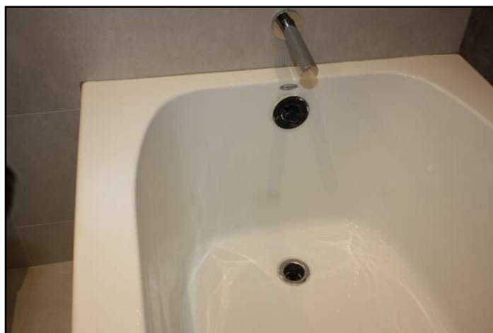
12. Overflows missing, leak, rust or...
