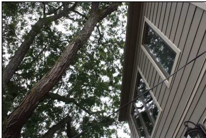
4. Trees or shrubs too close to building
