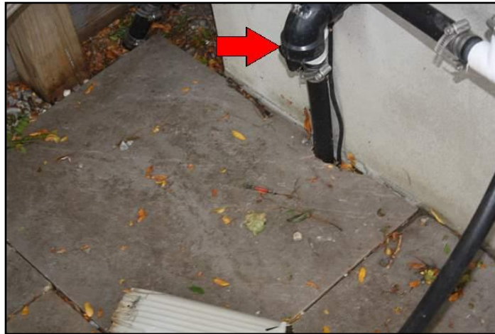
11. Discharge pipe problems
