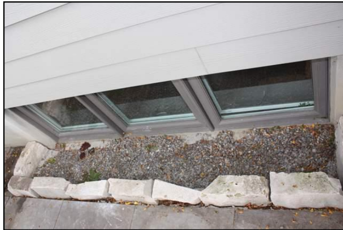
2. Window sill is at or below grade.
