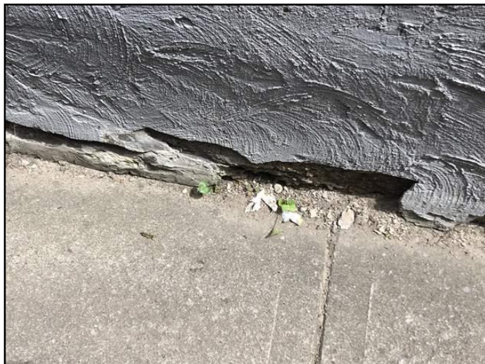
27. Parging damaged or missing
