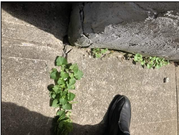
26. Parging damaged or missing
