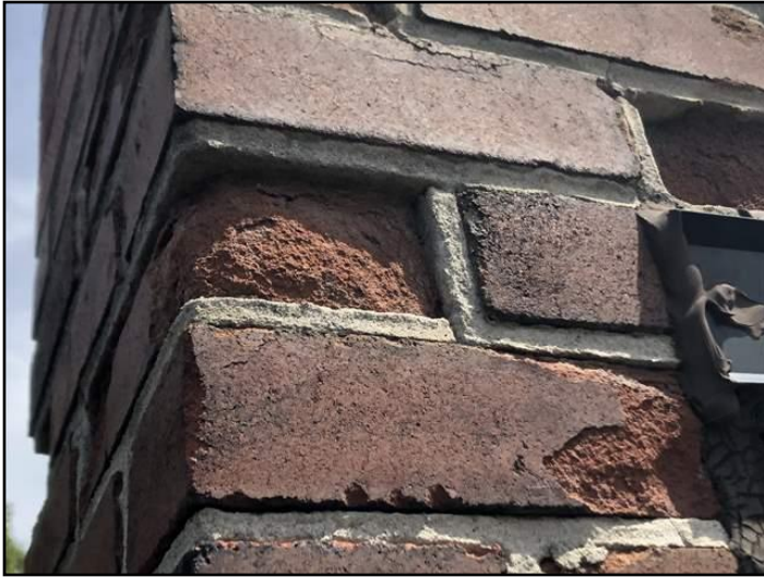
32. Loose, missing or deteriorated masonry
