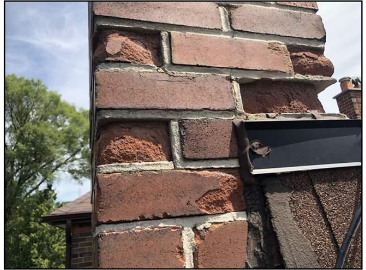
33. Loose, missing or deteriorated masonry
