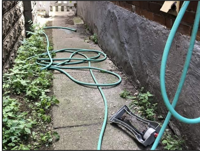
25. Improper slope or drainage
