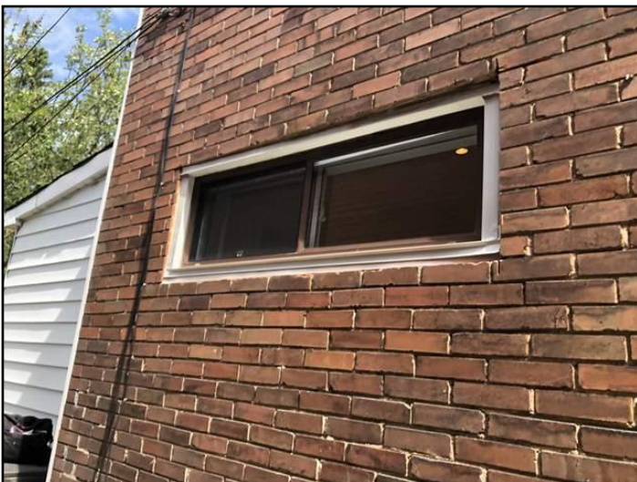
14. Flashing loose, missing or deteriorated
