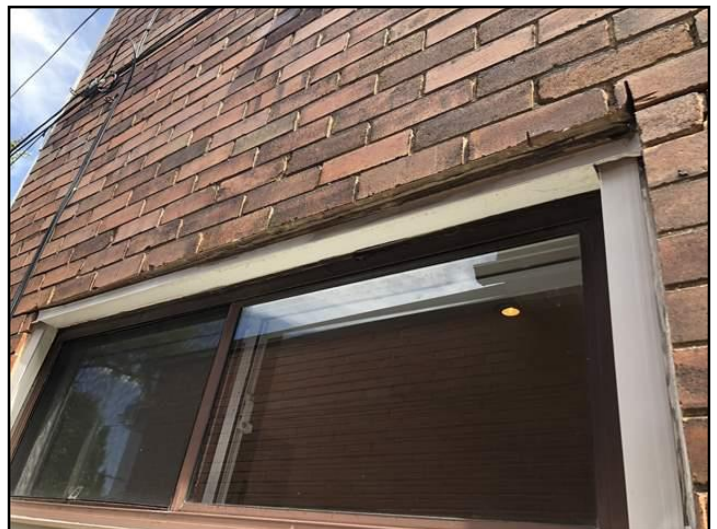
15. Flashing loose, missing or deteriorated
