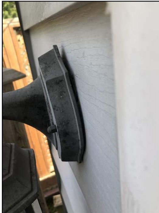
10. Caulking missing or ineffective
