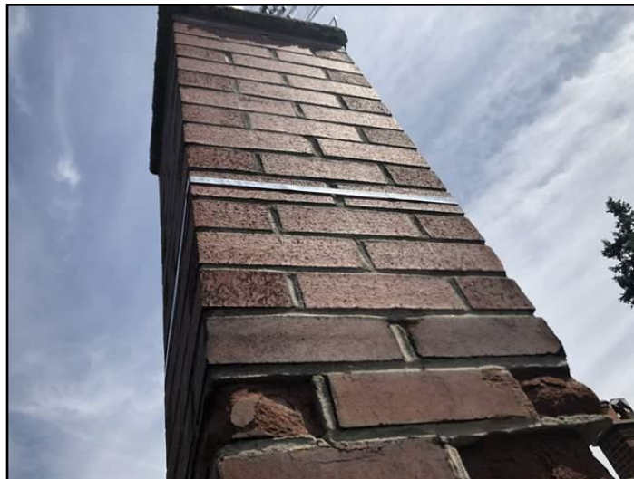
34. Loose, missing or deteriorated masonry
