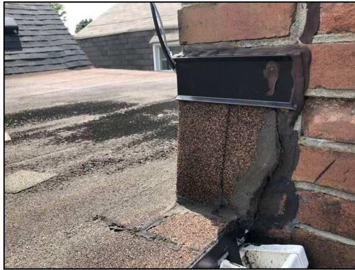
9. Caulking, sealant dried out, cracked
