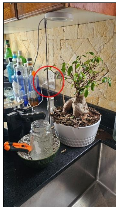
25. GFCI/GFI needed (Ground Fault Circuit...
