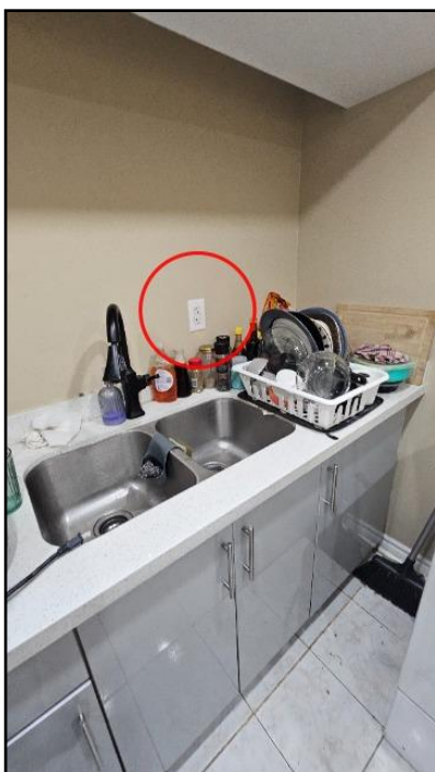
24. GFCI/GFI needed (Ground Fault Circuit...
