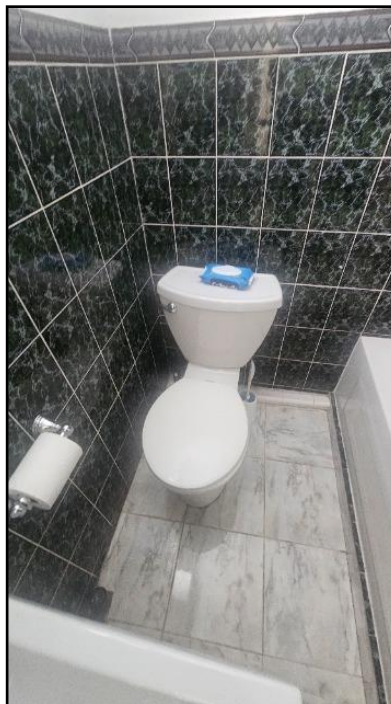
34. Loose Toilet Seat
